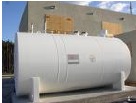
Double-wall above-ground storage tank
