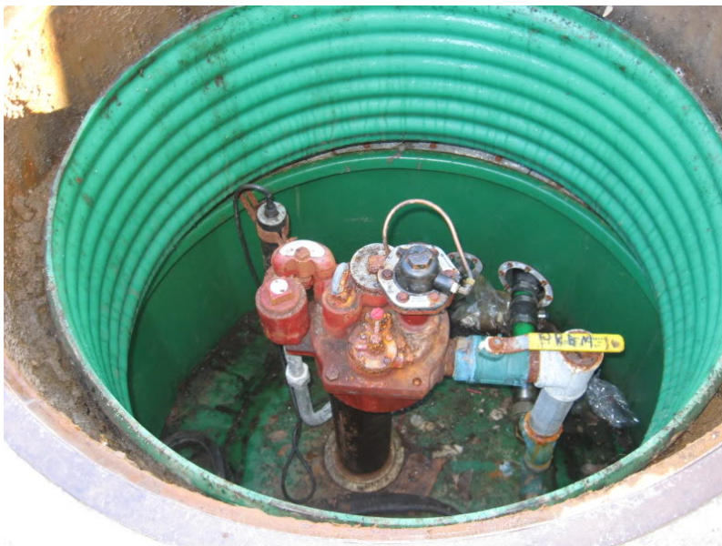
Sensor within a tank mounted piping sump
