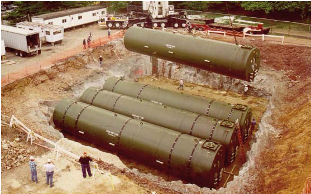
A typical UST installation
